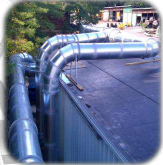
Dust Collection & Heavy-Duty Ducting Installed on Transportation Equipment Blast Room
