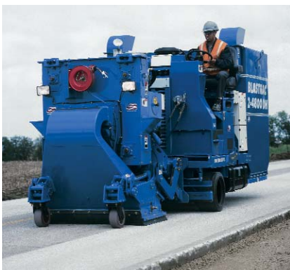
2-4800DH shot blast cleaning system
